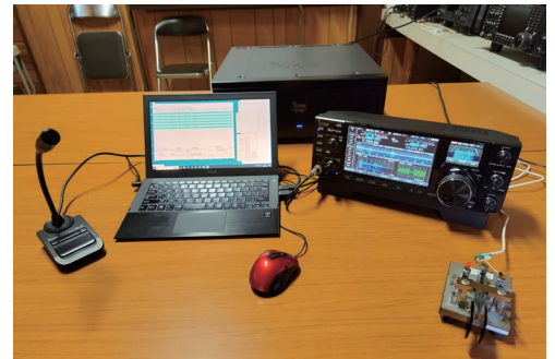
The Controller, PC, microphone, and CW paddle in front of the RF deck
